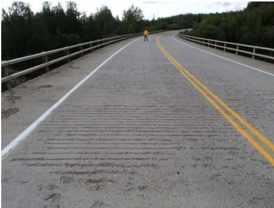
Figure 1: Damages on Chatanika River Bridge Deck
